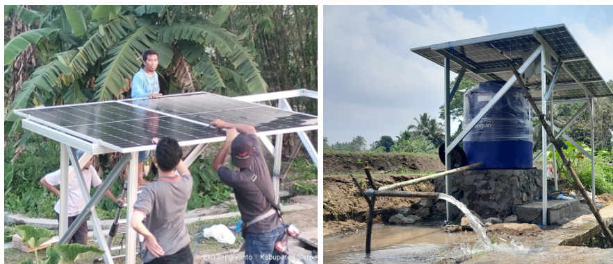
Gambar 6. Instalasi Pompa Air Tenaga Panel Surya
