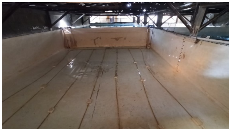
Gambar 1. Bak penampungan/ reservoir .
